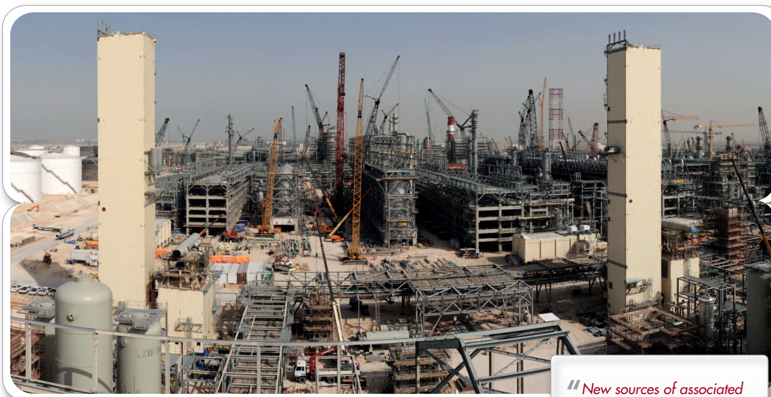
Gas processing associated with Shell's joint venture GTL project under construction in Qatar will result in additional ethane supply for petrochemicals production in the region.
