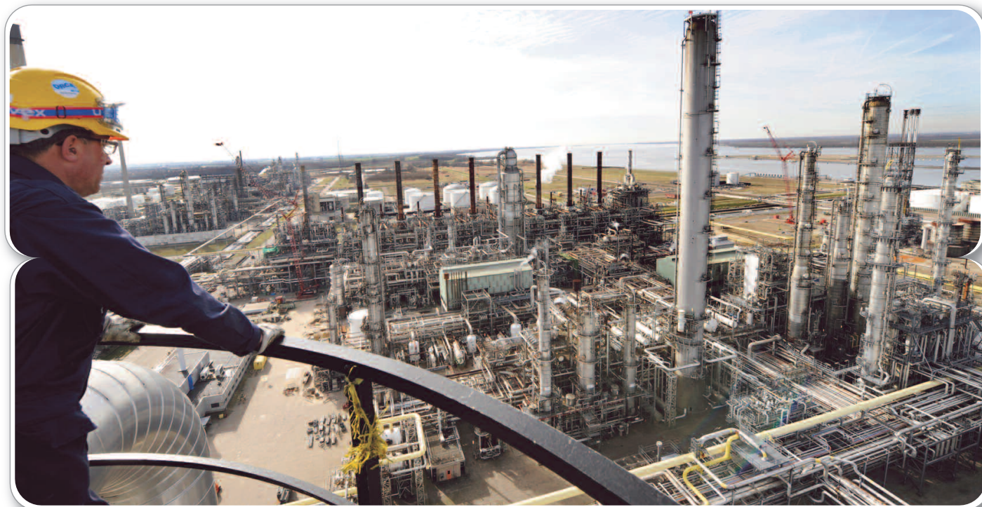
The CO2 prototype study at Moerdijk looked at every aspect of the site's operations that impact energy use and emissions.
