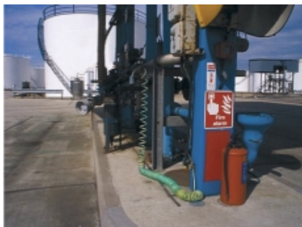
Typical truck loading area with grounding connection, fire extinguisher, and fire alarm switch
