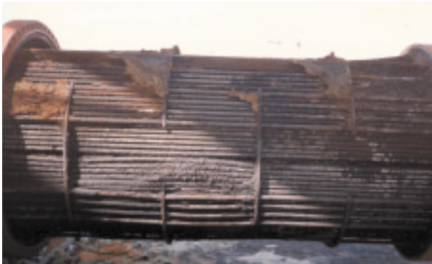
Fouling reduces heat transfer and increases pressure loss
