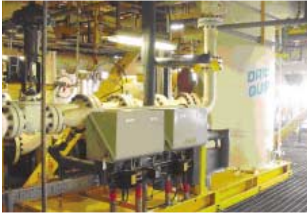
Slug suppression system for the Otter tie-back at the North Cormorant platform in the North Sea.
