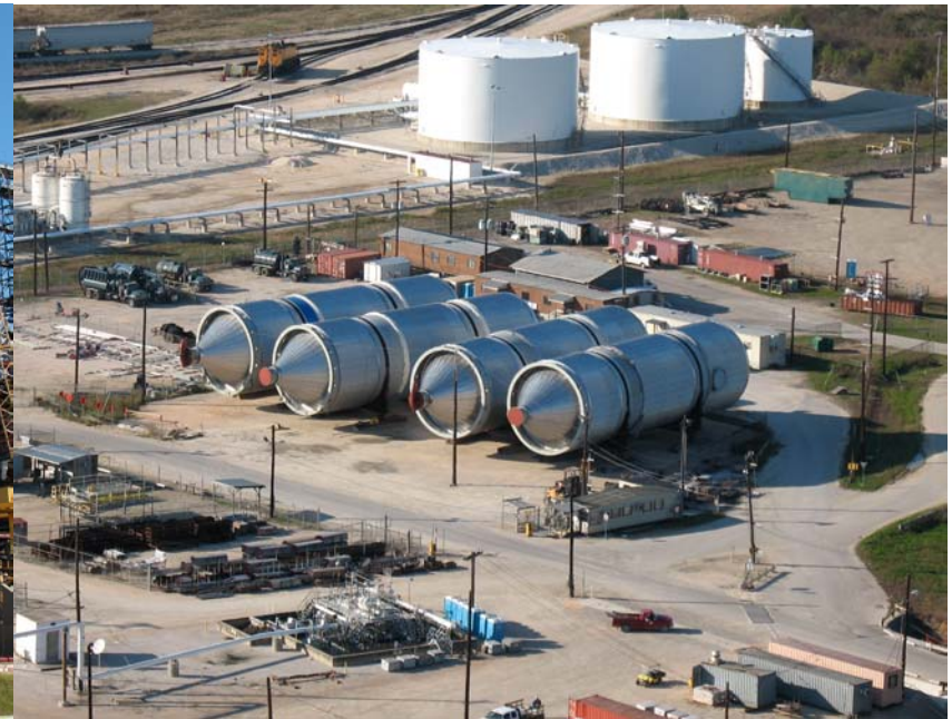
NEW COKE DRUMS
