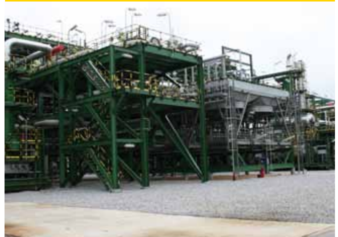
Dehydrating equipment – Gbaran Ubie
